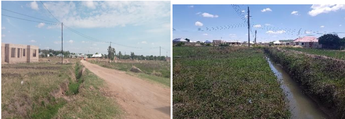
Figure 6.14: Siltation of the culvert and drainage structure at Kisarika I & IV road
