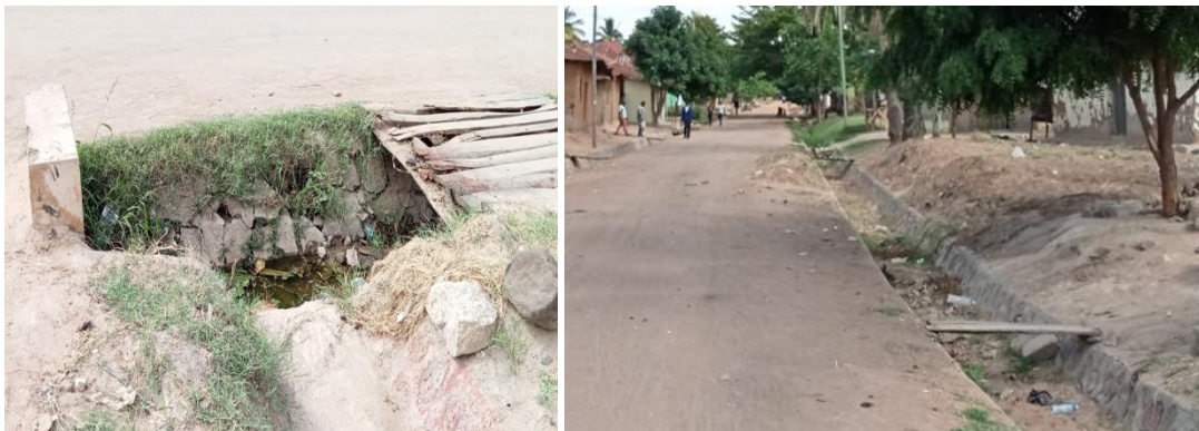
Figure 6.19: Siltation of the culvert and drainage structure at Kanyenye I&II road
