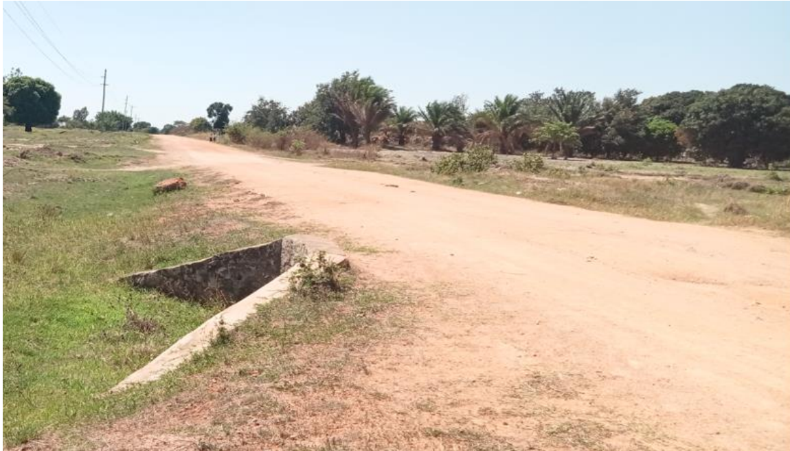
Figure 6.4: Siltation of the culvert and drainage structure at MailiTano road
